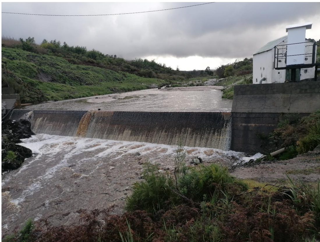
Figure 3-6: Weir G4H033 on the Onrus river, upstream of the de Bos dam inlet (20 July 2024).
