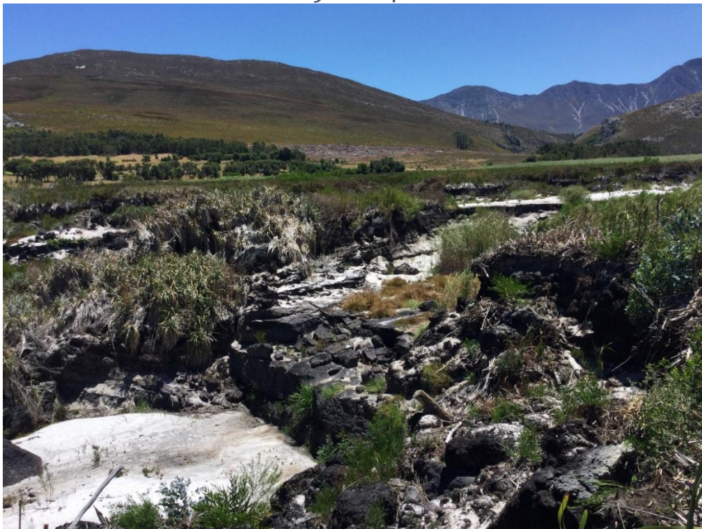
Figure 4.9 Extensive droughting of palmiet wetland as a result of gully erosion, leading to water table draw-down.
