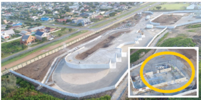
Materials-recovery and public drop-off facility currently under construction in Hermanus. The inset shows the location of the steel construction that caused the delay.
