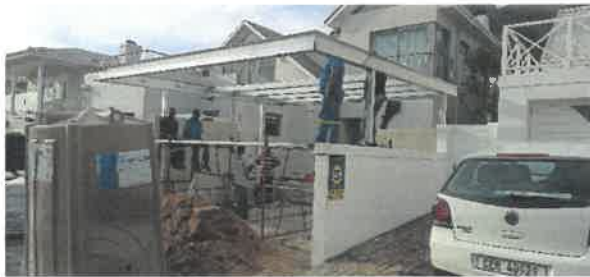
Image 3 (Indicating the upgrade of the carport on the 0m Street and 0m Common Boundary)
