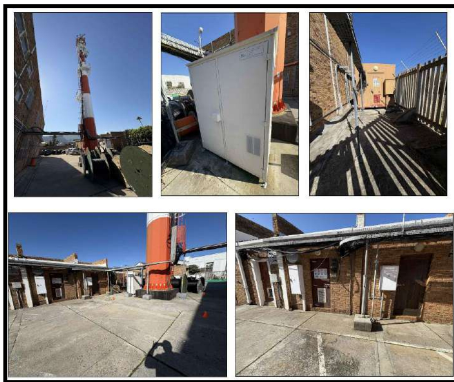
Figure 1 - Photos of the Existing Transmission Apparatus
