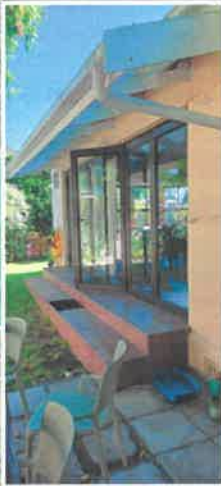
Awning exceeding the Northern and Northwestern Building Lines
