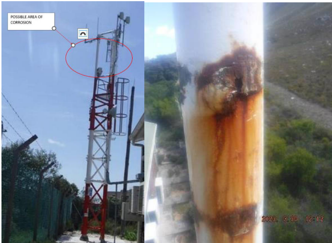
Figure 8 - Structural damage on the existing 10m Lattice Transmission Apparatus
