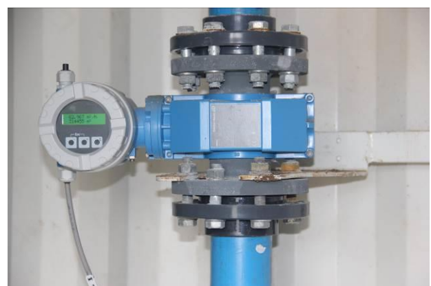
Stanford RO Plant (Filter feed meter)
