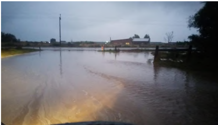
Figure 17: HEAVY RAIN CAUSED ROAD TO BE FLOODED AND ERODED THE ROADWAY AS WELL AS THE SIDEDRAINS
