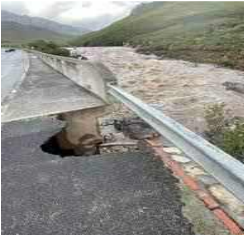
Figure 20: Flooding damage at Kleinmond bridge
