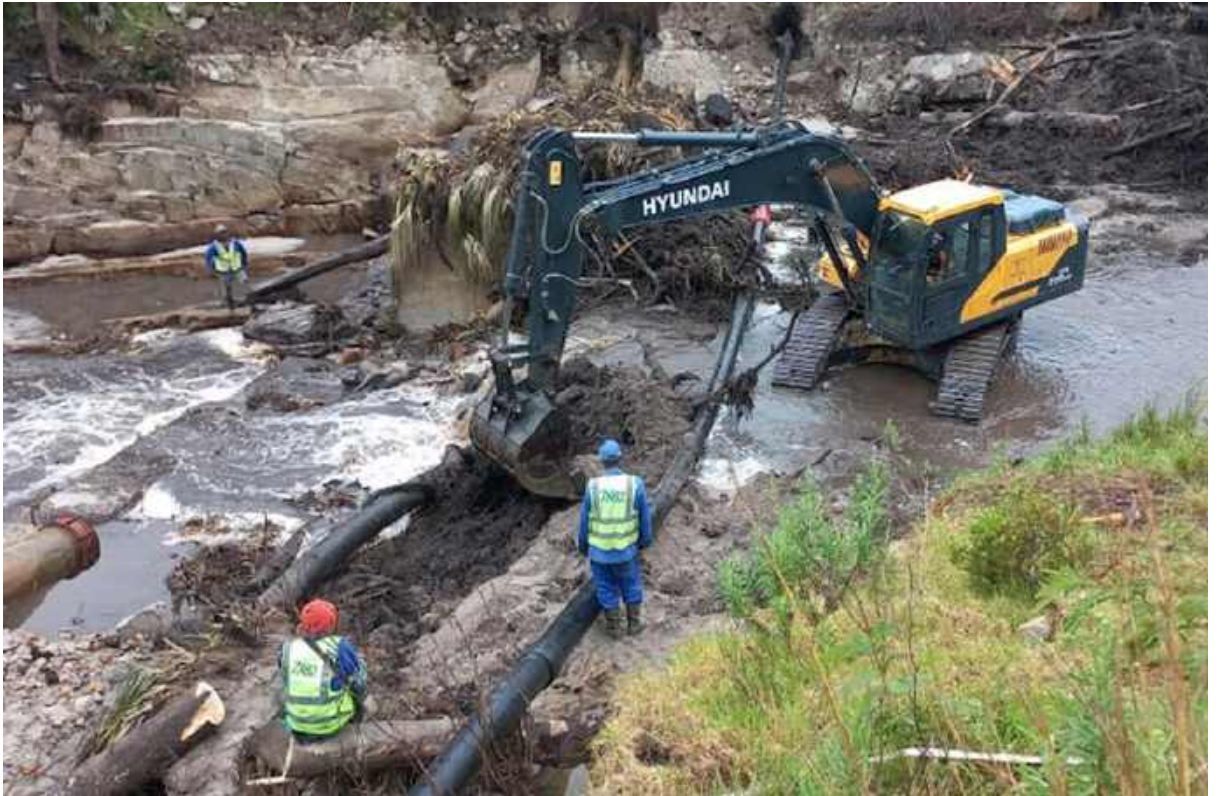
Figure 21: Pipeline repairs to damaged infrastructure
