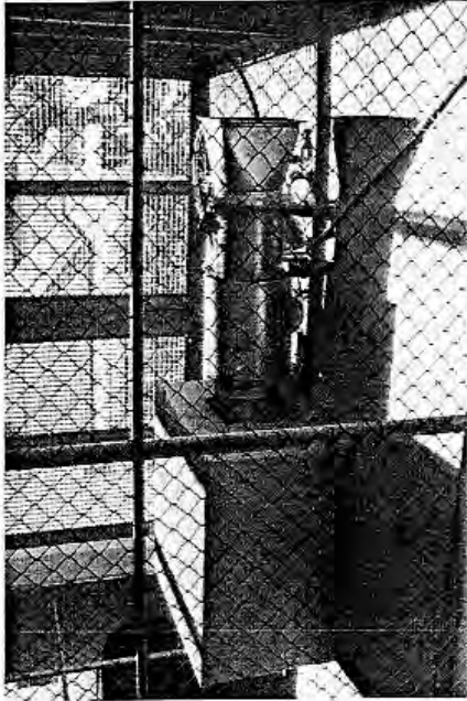
Photo 2 - 1st Floor fan
