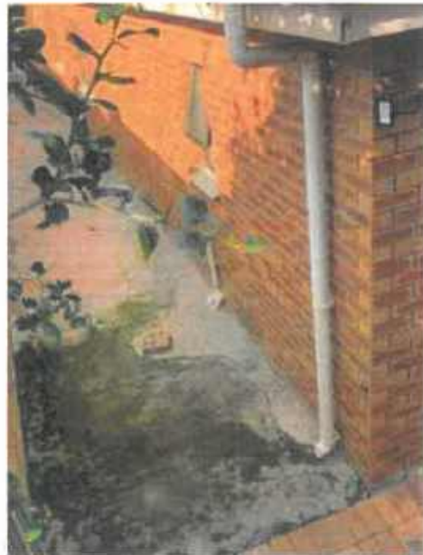
Mr. Hess's property where dampness is experienced.
