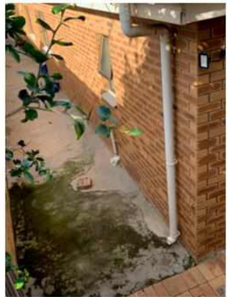
Mr. Hess's property where dampness is experienced.
