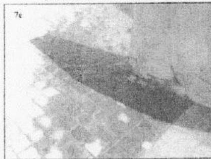
7e: Seepage at base of staircase to house and pool area.
