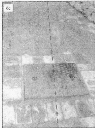
Manhole to pipeline carrying excess water from overflow inlet pipe in fish pond to the outlet at the bottom of the driveway.
