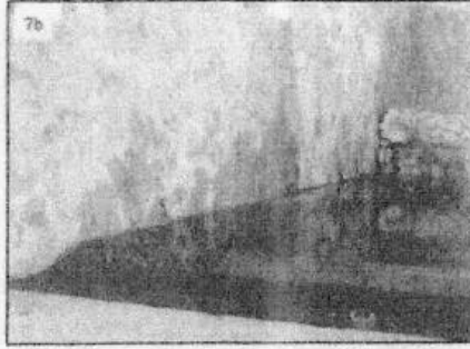
7b: Damp patches on stone-dressed retaining wall due to penetration of seepage water behind stone cladding.
