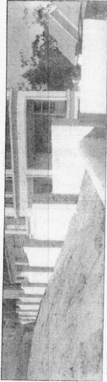
Neighbour's embankment above turning circle. Erosion resulted from stormwater flowing across neighbouring property and over their boundary wall.
