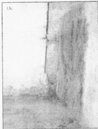
Staining of top surface of retaining wall where silt-contaminated seepage water emerges from voids in Mr Harper's wall.
