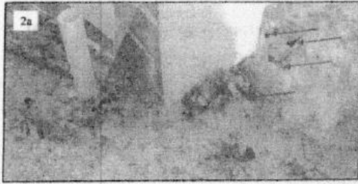
Voids at top south-east corner of retaining wall resulting from infiltration of surface water into backfill behind the corner column of this wall.
