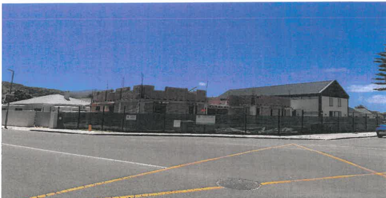
Building under construction at the corner of Aberdeen and Magnolia Streets. The structure occupies the corner position, with its footprint extending close to both street boundaries
