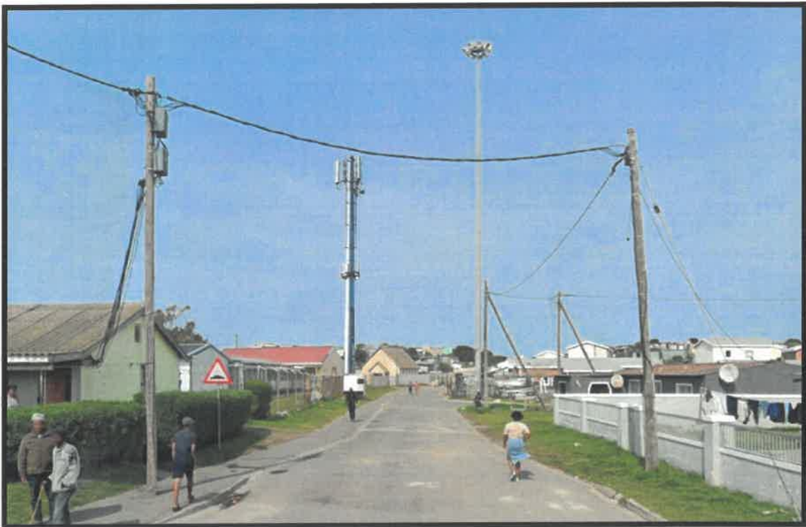
Figure 16 - 25m Monopole mast viewed from Hlobo Street
