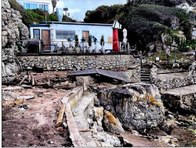
(Figure 2 depicting the damage of the September 2024 storm event with the wooden decks, furniture and balustrade completely destroyed)
