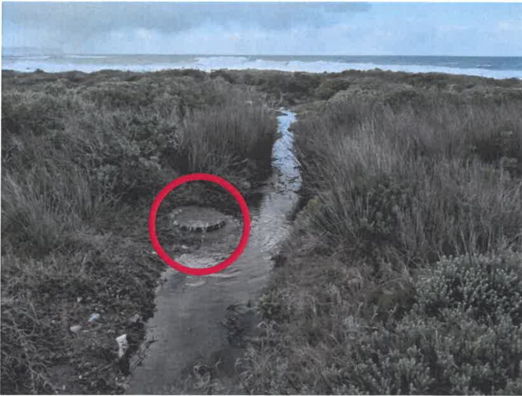
Figure 4 Note the excess water spillage from a sewer line during a downpour
