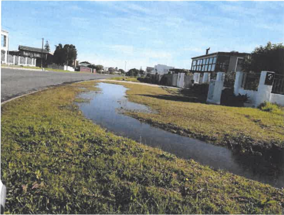
Figure 2 Indicating a lack of rain water drainage on the eastern side of Main road
