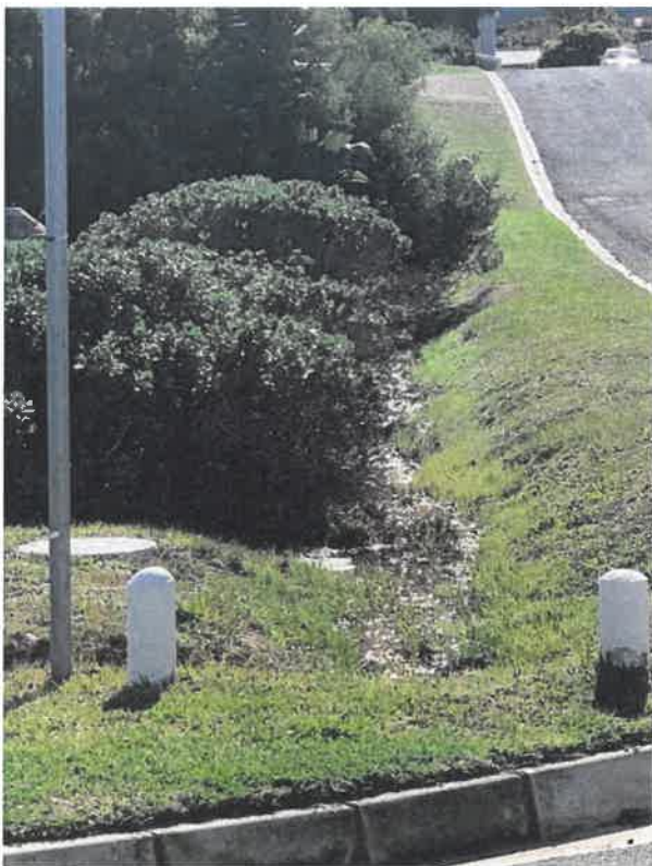
Figure 7 A typical example of a water gully in Sandbaai that is overgrown with vegetation
