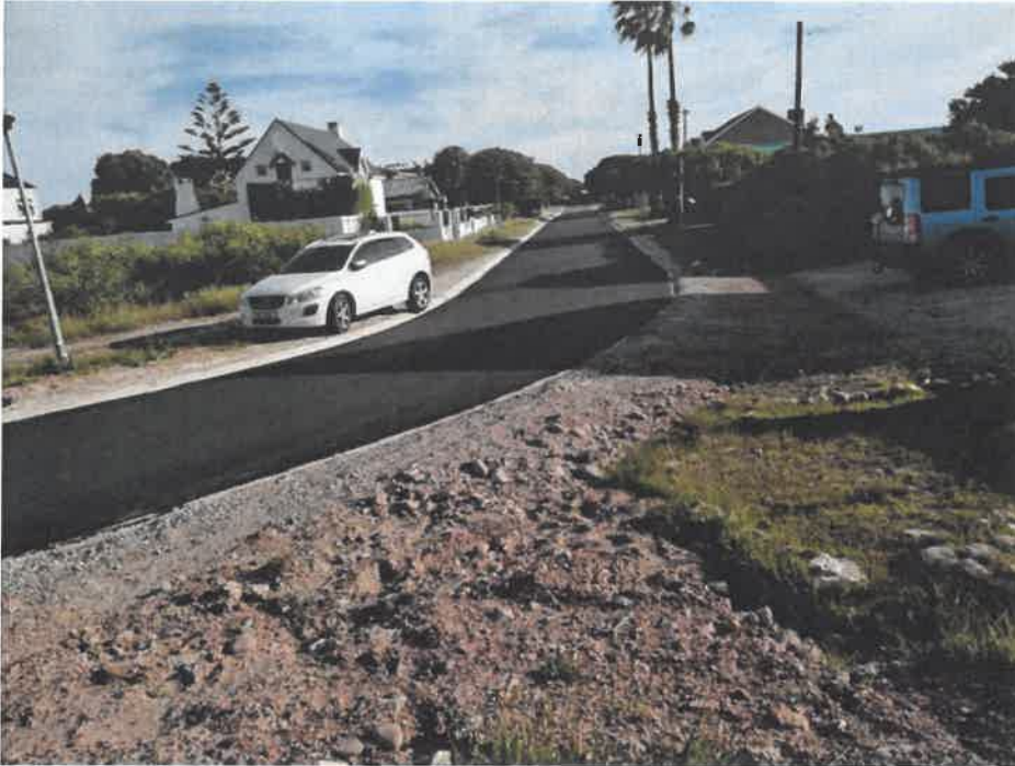
Figure 12 After a successful intervention and re-engineering of the water flow the problem was solved
