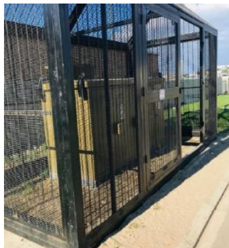
Safe gurading of eletrical transformer (Ward 6)
