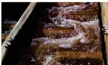
Cascading Inlet for conventional treatment - Preekstoel WTW
