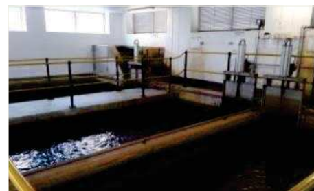
Biofiltration Plant - Preekstoel WTW
