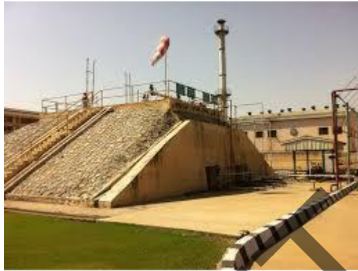
Example of a mounded tank facility
