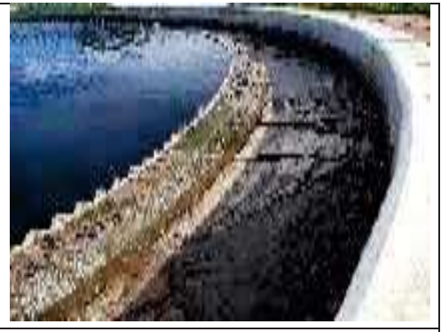
Flow distribution uneven and deliver high flows to 1 of 4 clarifiers. Work done during TSA to rectify this design defect.
