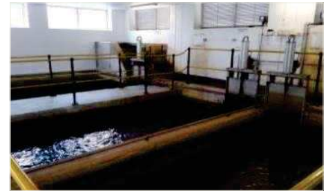
Biofiltration Plant - Preekstoel WTW
