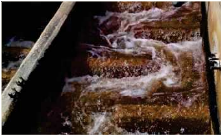
Cascading Inlet for conventional treatment - Preekstoel WTW
