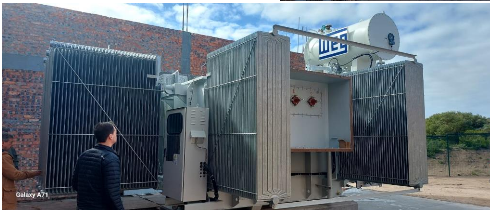
Birkenhead 66KV Substation and Overhead lines
