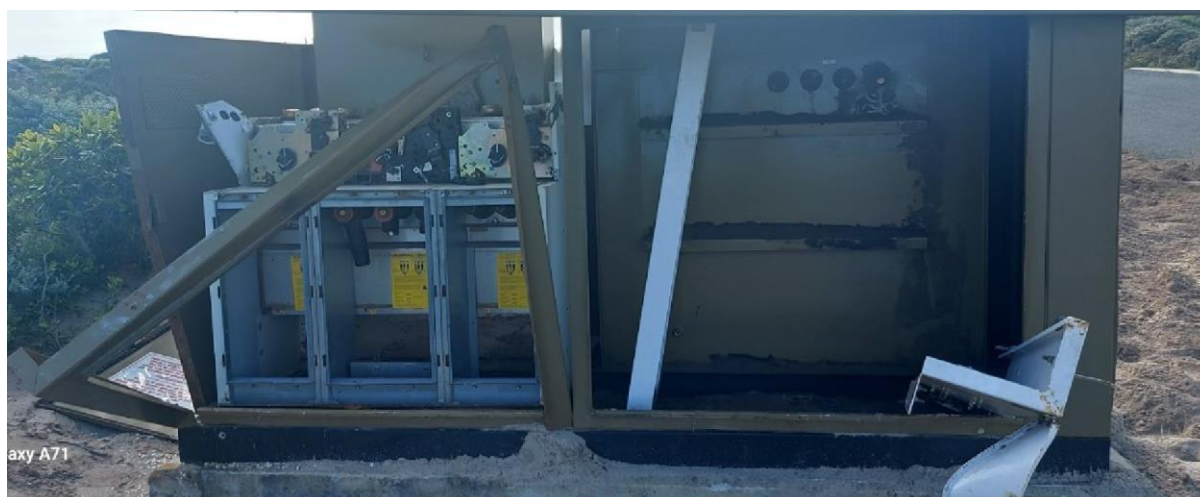
Theft and Vandalism of Electrical Infrastructure
