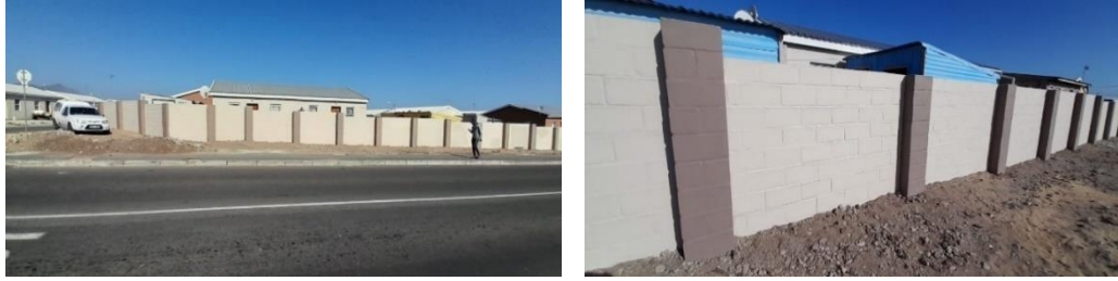
Site C1 & C2, Swartdam Road – Boundary Wall
